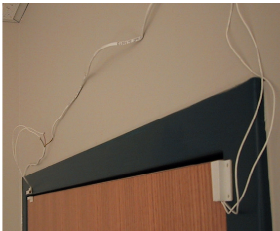
Figure 9. A photograph showing two magnetic contact-switches affixed to a door. The placement was chosen to discriminate between the open and ajar door states.
